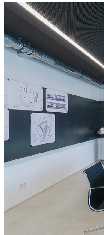
The flush installed SLOTLIGHT strip light in the conference room accommodates the form of the conference table.
