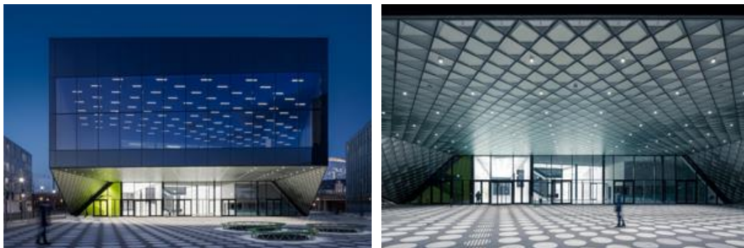
Fig. 7 + 8: The lighting extends into the outdoor area with a series of OPTOS downlights. These are mounted in cast-glass façade cassettes in the ceiling, forming a continuous connected interactive light matrix that covers the entire ceiling canopy.
